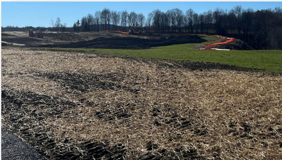
Town of Florida (Montgomery County): Topsoil storage and protection on solar array.
